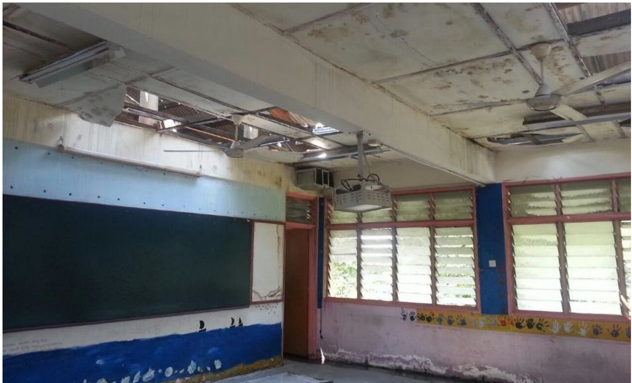
Ceiling of the school falling down presenting a hazard to students and teachers.
